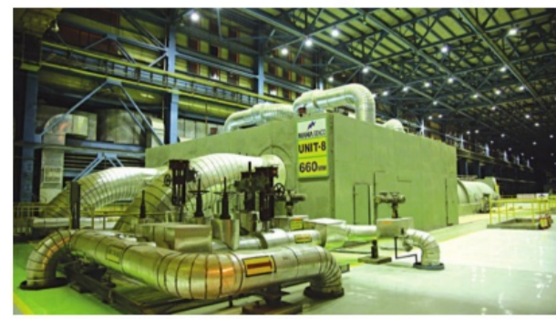
units in Paras, Khaperkheda and Koradi, and ESP retrofitting work at two Chandrapur 500 MW units is in progress.
